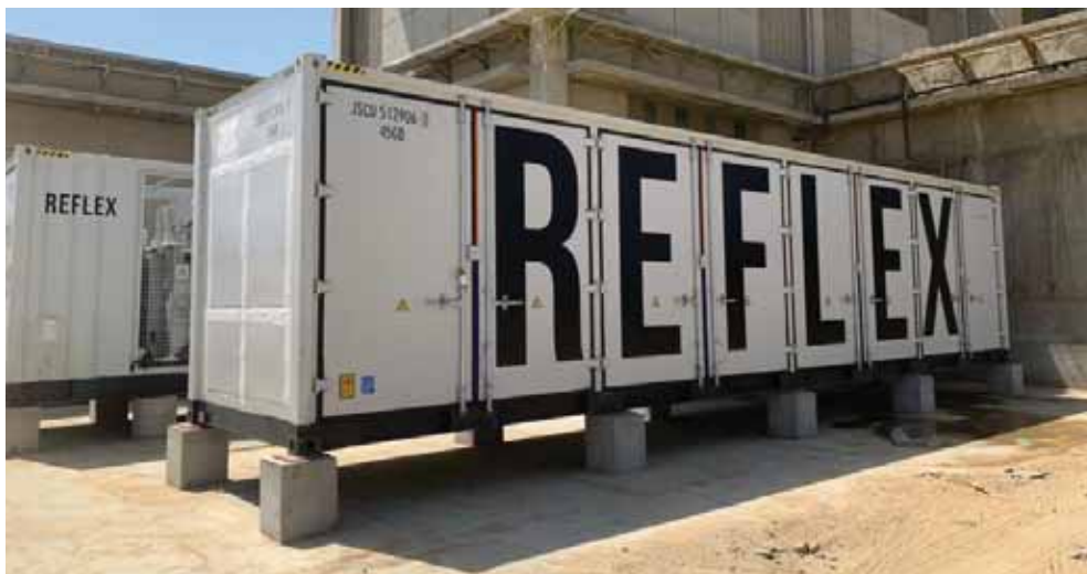
BESS system at Gatron (Industries) Limited
